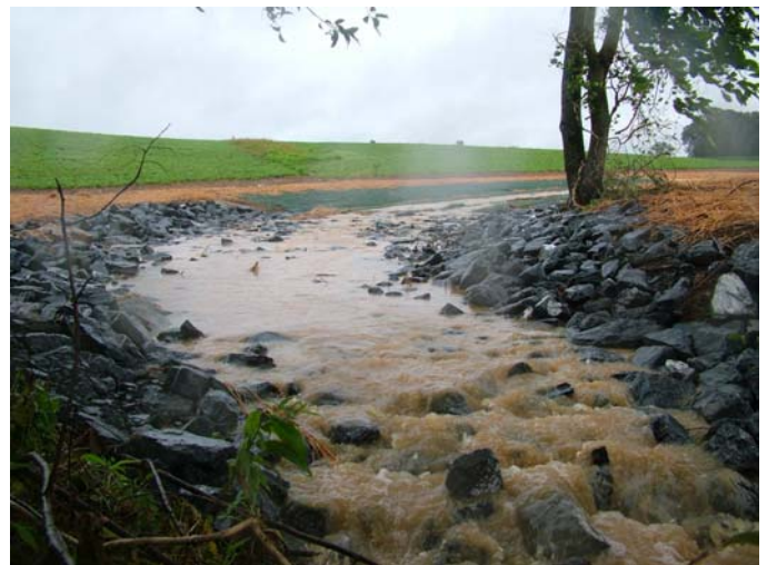
Stone rip-rap outlet for a waterway.
